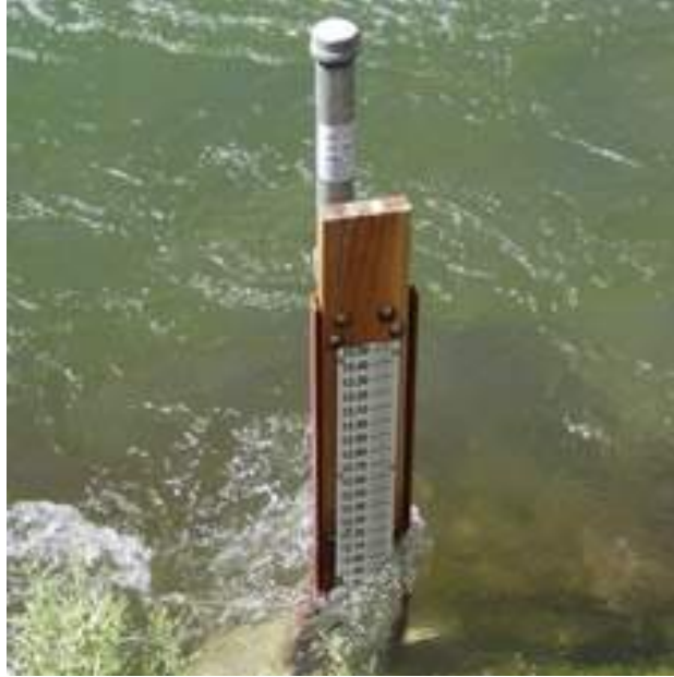
Figure 6 – Simple Stilling Well and Staff Gage Setup
